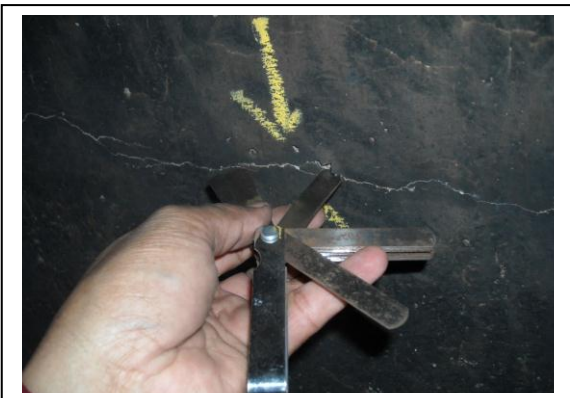
Gambar 2. Retak garis arah circumferential
